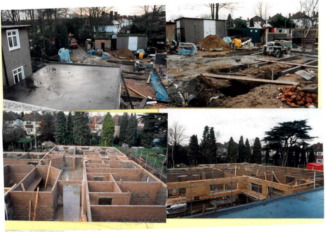
Foundations being laid for the new wing of the Inpatient Unit at John Taylor Hospice 1994
